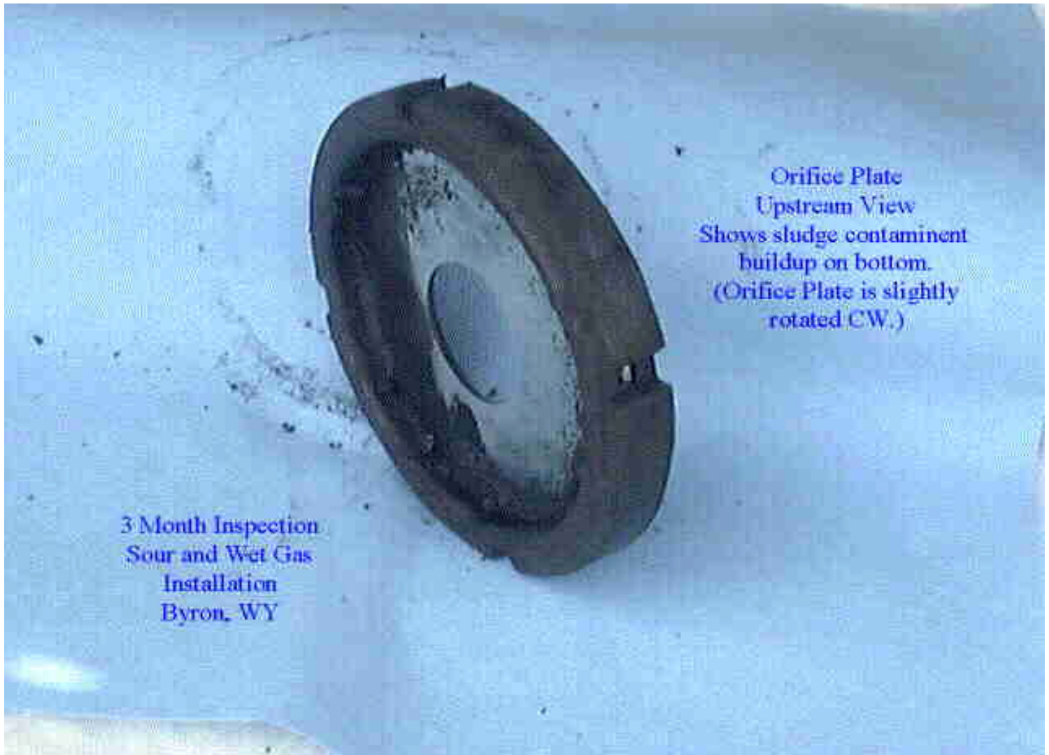
Three months inspection for wet gas line (H 2 s + paraffin's)
